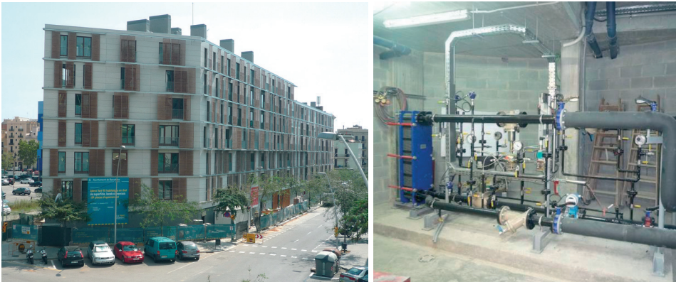
Figure 17: Some 95 apartments connected to district energy in Barcelona Innovation District 22@. (Source: SaAS)
