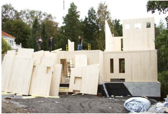
Erecting a house made of prefabricated solid wood elements in Pispala, Tampere.
